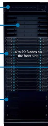
42U cabinet front view
